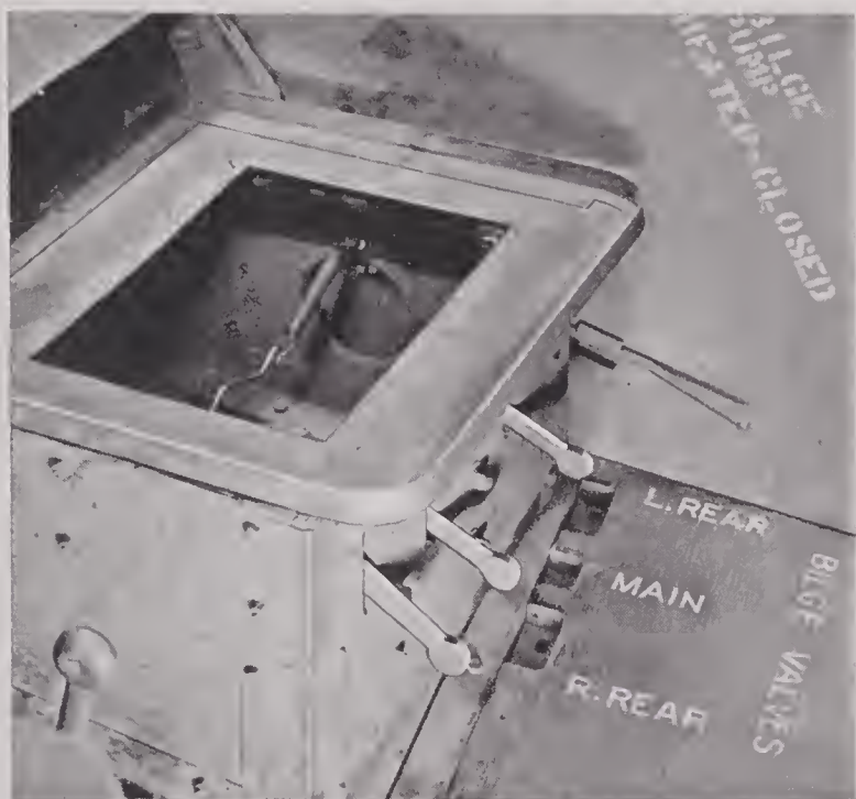
FIGURE 18. Manual controls for bilge pump manifold.
